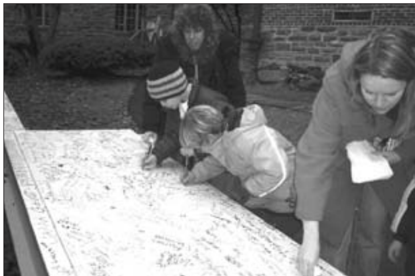
On January 6 the final beam for the new middle school was hoisted into place. Earlier in the week, Fieldston Lower students were among those signing the beam.
