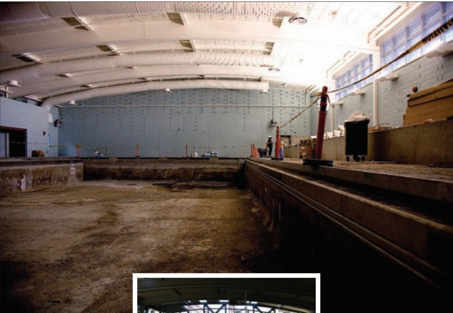
September 2006: The new pool nears completion. Right: September 2005, framework goes up on the pool building.
