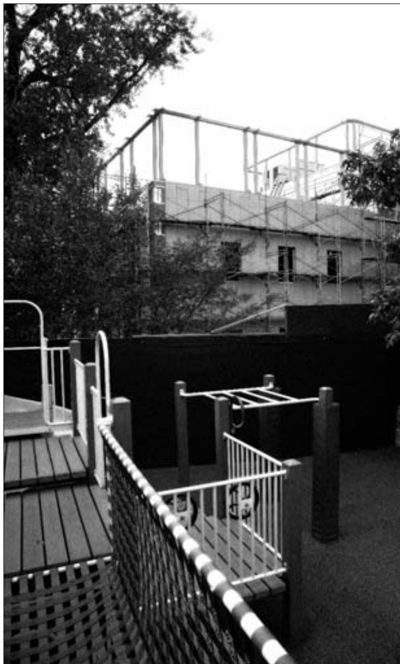
A view of the new middle school building from the Fieldston Lower playground.
